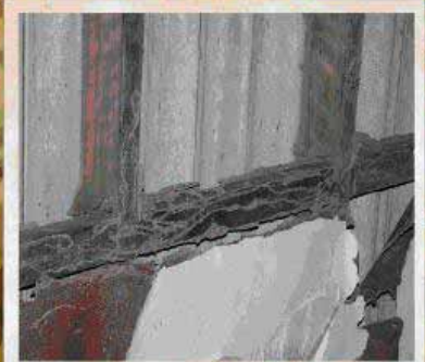
Mud trails in buildings and trees are evidence of giant termite activity
