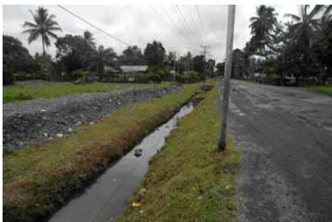
Figure 10. One of the deep drains which are thought to be limiting spread of the termites.
