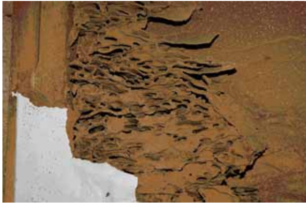
Figure 11. Damage at the Police Barracks.
