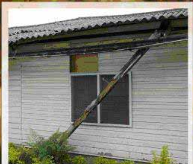
The exterior of a building destroyed by giant termites
