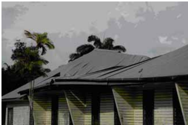
Figure 3. The SDA church which was damaged when a large tree killed by termites fell.
