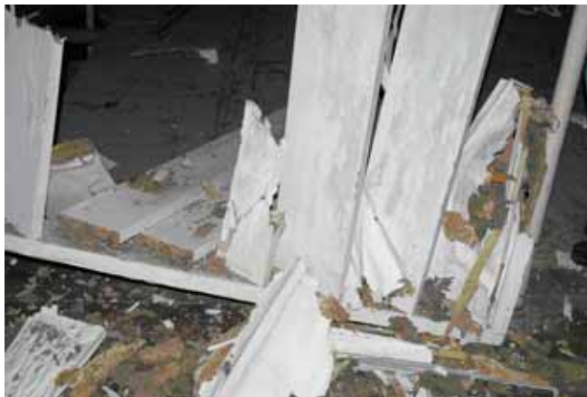
Figure 4. Damage in the hospital.
