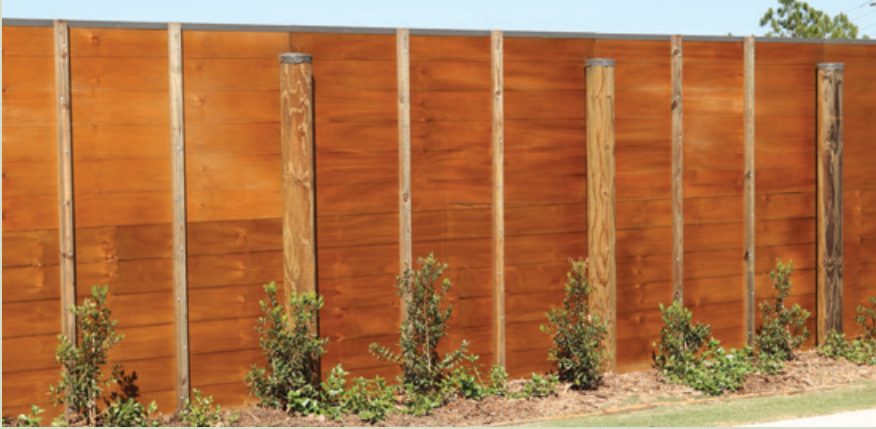
Figure 2.4. A plywood noise barrier.
