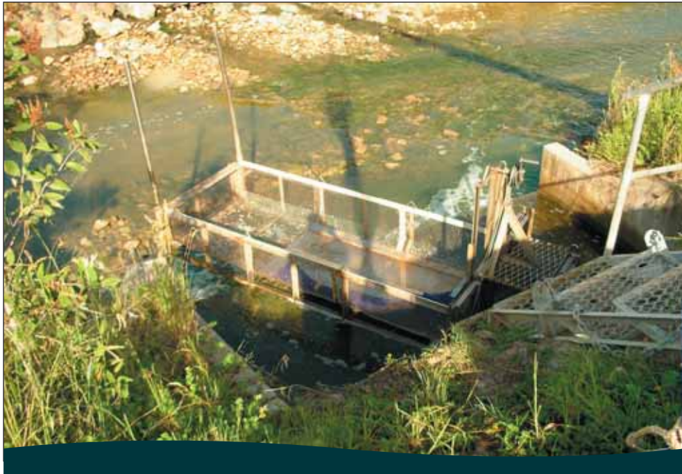
Figure 2.9 Harvest cage installed at the pond outlet
