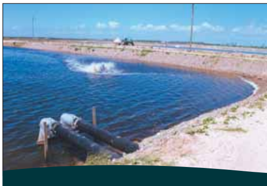
Figure 4.4 Filter screens or 'socks' installed on pond outlet pipes
