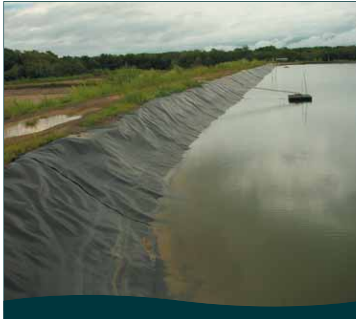
Figure 2.2 HDPE black plastic liner installed on a pond wall to minimise erosion from wind action and rain
