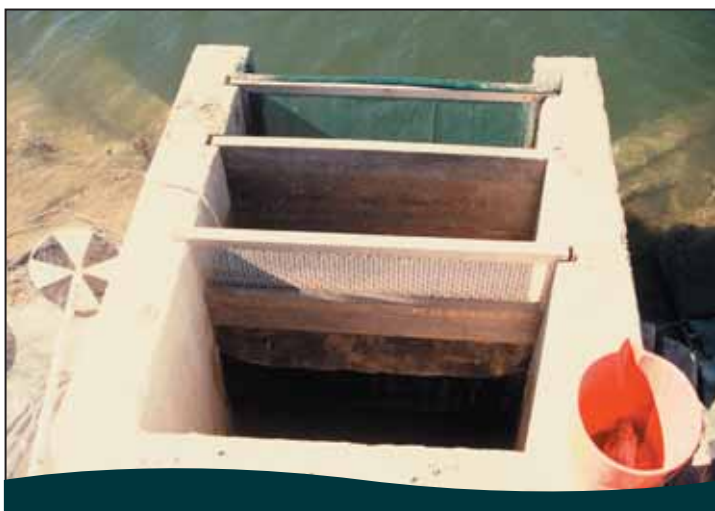
Figure 2.4 A 'monk' water control and outlet structure
